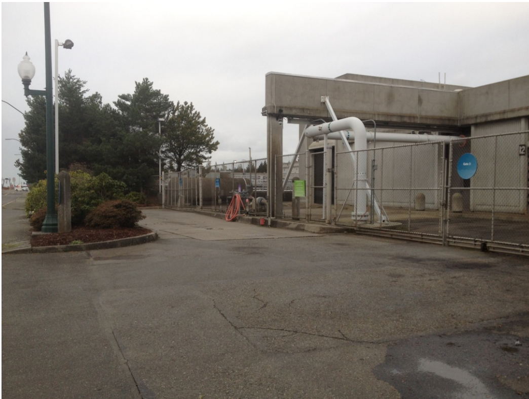
Figure 4-4. Septage Receiving Station
