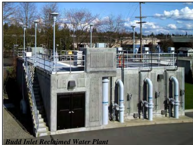
Budd Inlet Reclaimed Water Plant
