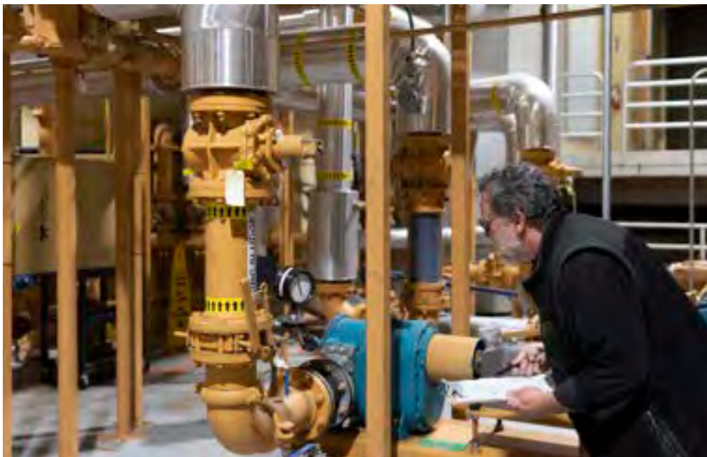
The Digester System Improvements project includes refurbishment of aging components associated with the sludge digestion system.
