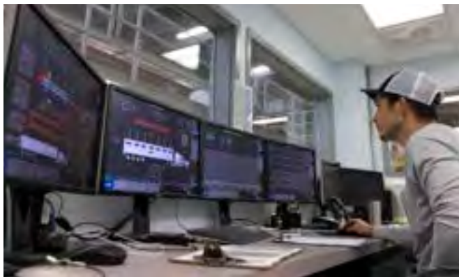
LOTT operates its treatment facilities continuously to ensure that wastewater is properly treated and cleaned before it is released into the environment.
