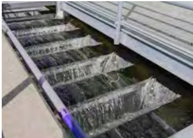
LOTT treats an average of 12 million gallons of wastewater each day.
