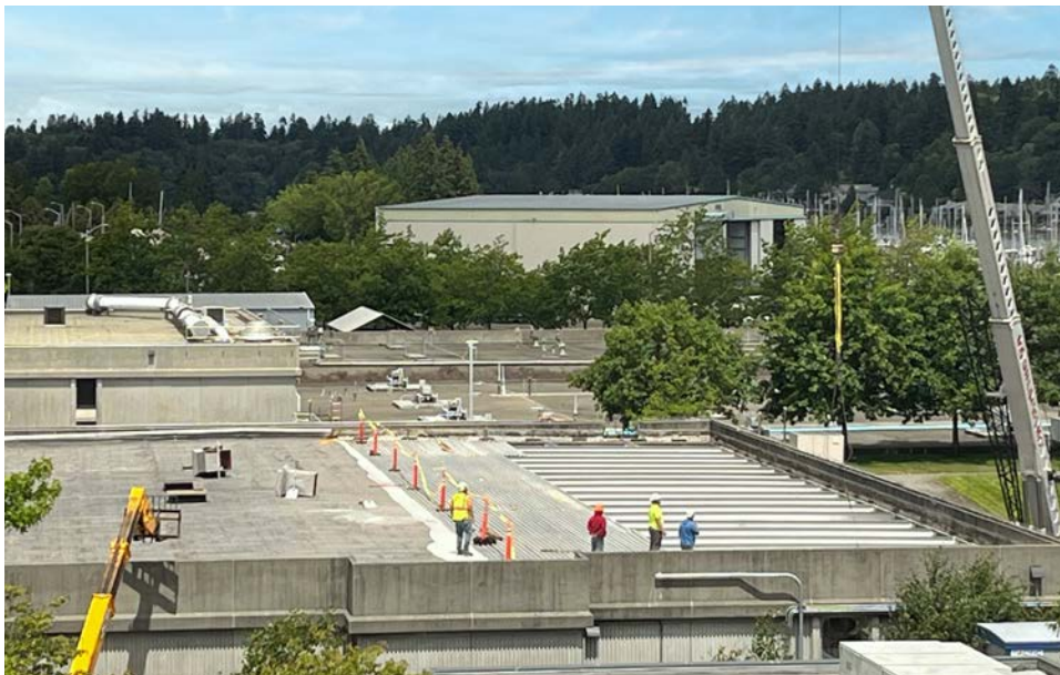
The projects identified in the CIP are necessary to ensure LOTT sustains the existing wastewater treatment system and provides needed new system capacity.
